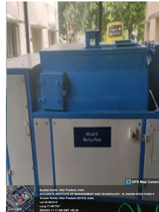
BIO GAS PLANT NEAR HOSTEL-2
