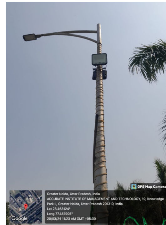
LED STREET LIGHT IN CAMPUS
